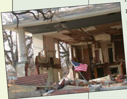
ABOVE: Hurricane Katrina gutted this house east of Gulfport and west of Biloxi, Miss. The second-floor structure is missing. Note the second-floor fireplace on the upper left wall.
